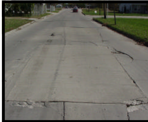
Example of condition of the pavement replaced as a result of this project
