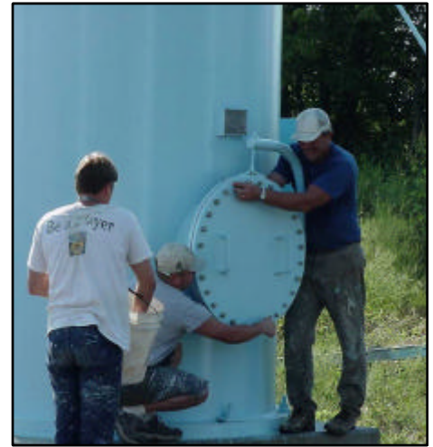
Securing of the bottom Manway prior to disinfection and filling to put completed tank in service
