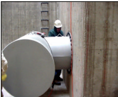
Filter screen bolted in place
